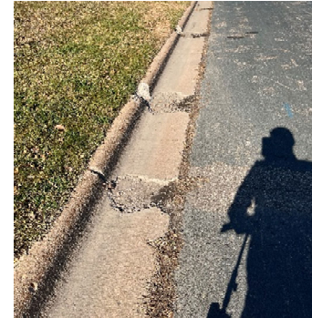
Existing curb joint failure
