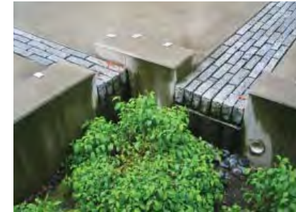
Water collection systems integrated into pavement areas
