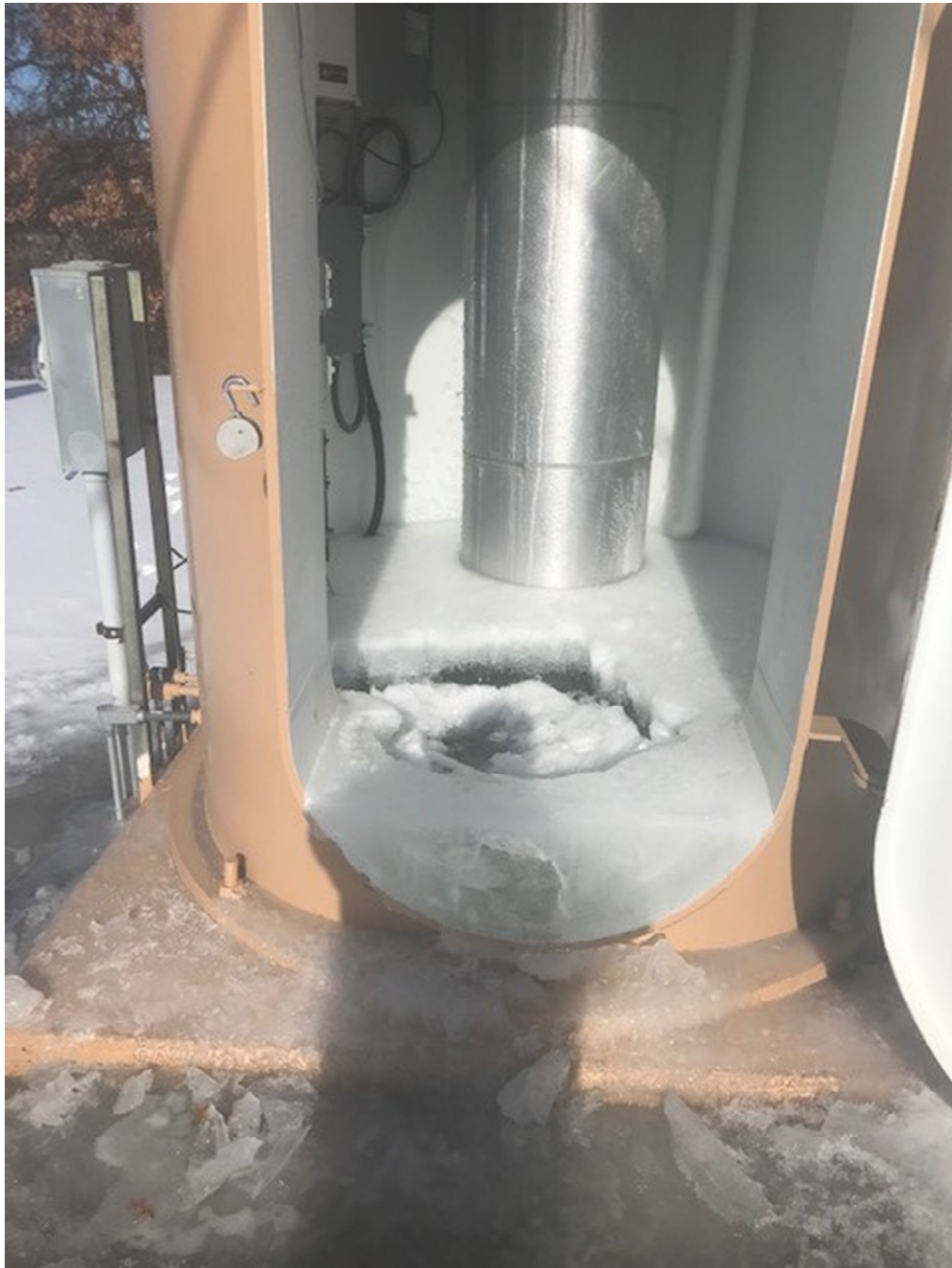
Photo No. 1 View of dry riser base after developing leak in winter 2022
