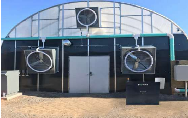
Greenhouse with ecosorb system installed near rear fans
