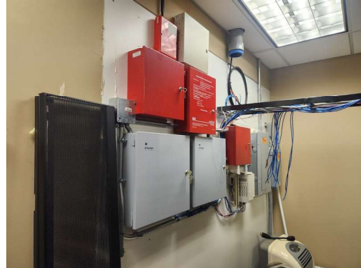
28. Fire alarm system
