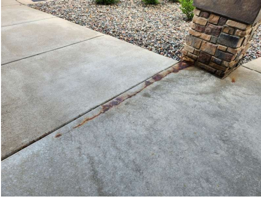
13. Cracking and stained concrete
