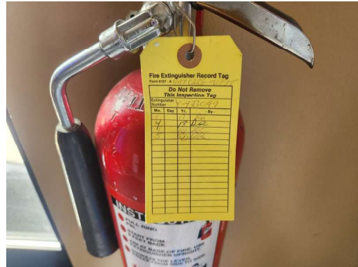
34. Fire extinguisher (expired)
