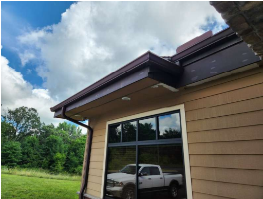
15. Peeling paint under eave
