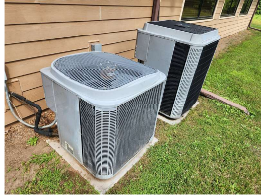
20. Air conditioning units
