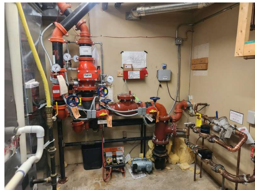
30. Fire suppression system
