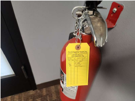
33. Fire extinguisher (expired)
