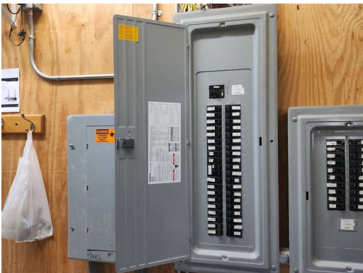
29. Typical electrical panels
