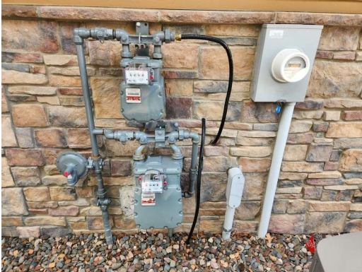
21. Gas main and meters
