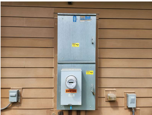
17. Main power connection
