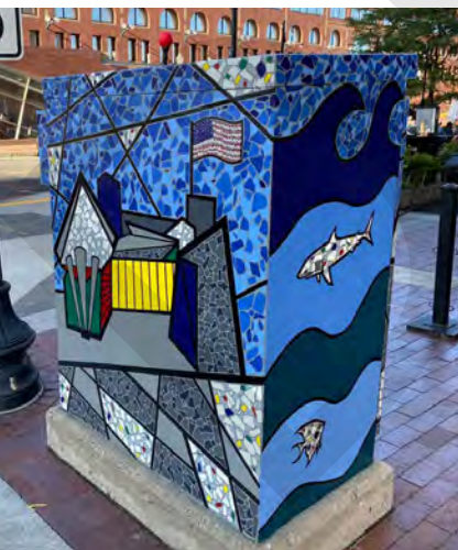
Example: Painted electrical box.
