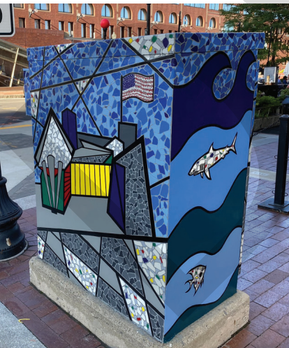
Example: Painted electrical box.
